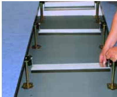
2. Mounting of the carrier profiles for the application of the insulating heating units.
