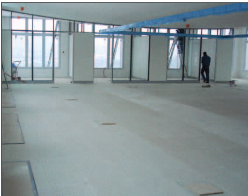
Barmenia Office Building - MERO hollow floor Combi T
